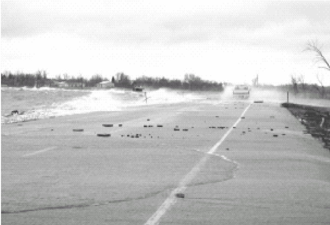
Figure 2. Waves crashing over LIS Highway 281 in 2004. This highway has been rerouted to the west to prevent repeated problems with waves eroding the road.
